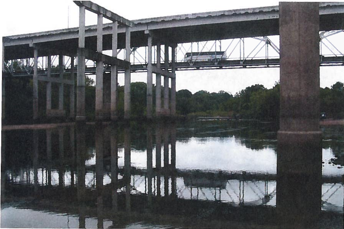
View of existing structures at project site – note bridge column in foreground of existing northbound bridge; existing bridge columns in place for future northbound mainlane bridge; deck and columns of existing southbound bridge; and existing truss bridge carrying southbound traffic from on-ramp.
