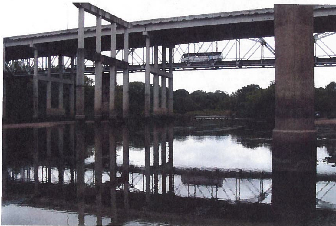
View of existing structures at project site – note bridge column in foreground of existing northbound bridge; existing bridge columns in place for future northbound mainlane bridge; deck and columns of existing southbound bridge; and existing truss bridge carrying southbound traffic from on-ramp.
