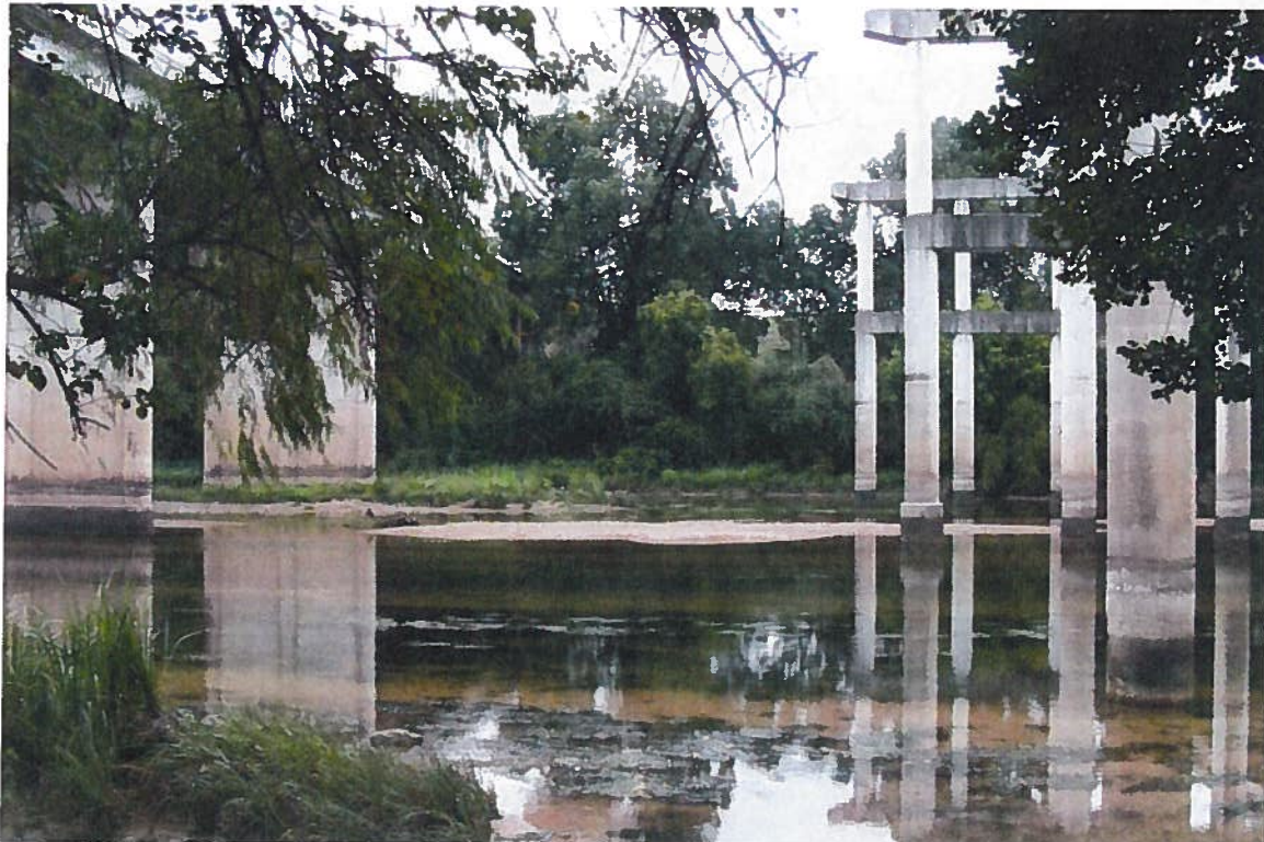
Proposed Northbound Exit to Airport Blvd bridge to be added to existing northbound mainlane (NBML) bridge on left. View from north to south bank.
