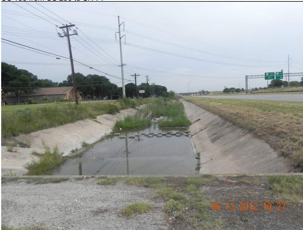
Carson Creek: Standing west of US 183 looking north at concrete lined channel south of the interchange with SH 71.
